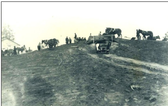
Construction of a levee in Elba, Ala., in 1933 or 1934. Levees were constructed in several areas around the state to control flooding.
